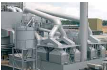
Flue gas purification in the power industry. State of the art filter processes and systems for removal of pollutant gases.
