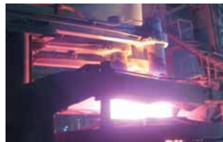
Dust collectors for electric arc furnaces in steel plants with accessories such as coolers and spark arrestors.
